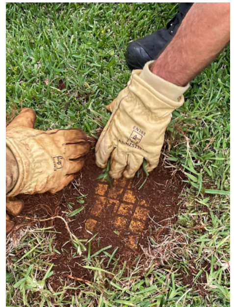
Covered hydrants hamper rescue efforts Photo supplied
