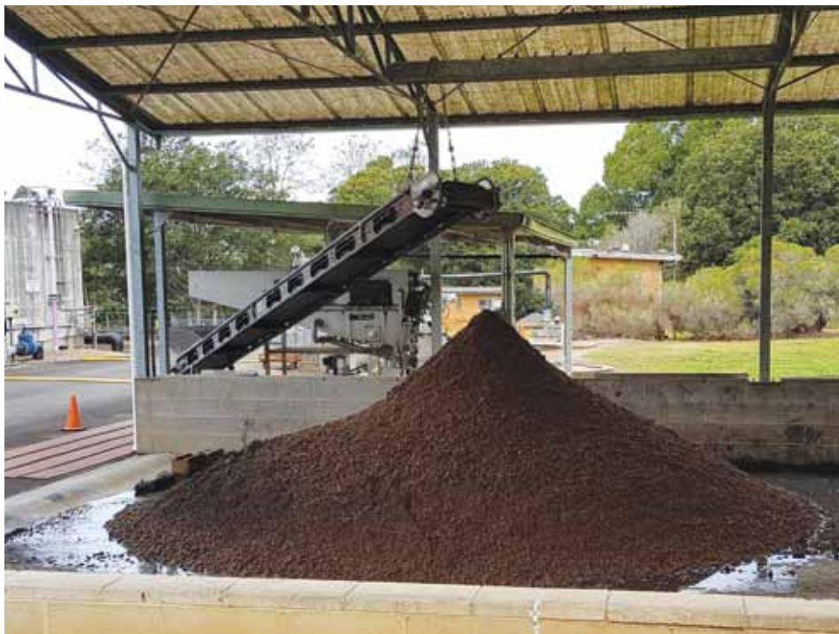
STP processing plant
